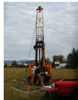
Buckley Substation Site
